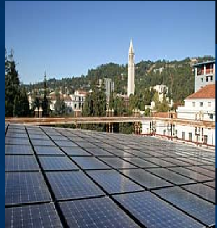
UC Berkeley's 120 kW PV array, located on Martin Luther King Student Center roof
